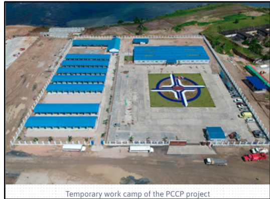
Temporary work camp of the PCCP project Image 5.4.1.2: Screenshot and caption of "work camp" from port website
