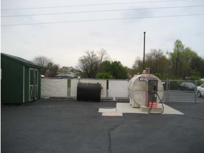
ABOVE GROUND GASOLINE STORAGE TANK
