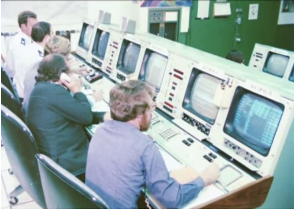
Figure 34. The console configuration within the Satellite Test Center evokes images of other control centers, namely NASA's Mission Control Center. Source: "Air Force Satellite Control Facility," by Space and Missile Systems Center, Los Angeles AFB YouTube user, estimated 1980, https://www.youtube.com/watch?v=ZX9cq3_vgkI
