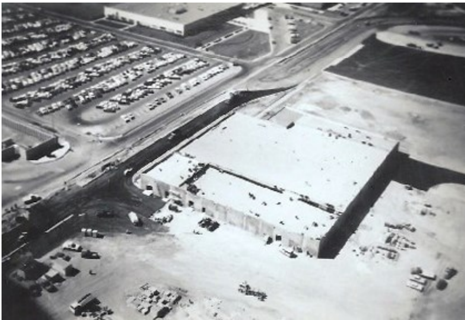
Figure 32. An aerial view of Building 1001 in 1959 shows the beginnings of what would become a large complex. Source: Onizuka AFS
