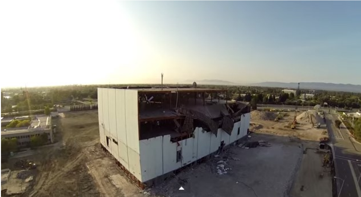
Figure 39. The Blue Cube was demolished in 2014. This still was taken from a video captured by a private UAV equipped with a GoPro. Source: "Goodbye Blue Cube, Sunnyvale, CA," https://www.youtube.com/watch?v=YOmb49SQ-x4
