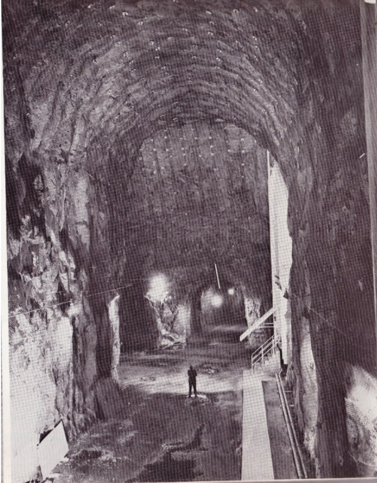
Figure 22. The excavated mountain interior. Source: Henry W. Hough, NORAD Command Post: The City Inside of Cheyenne Mountain (Denver, CO: Green Mountain Press, 1970).
