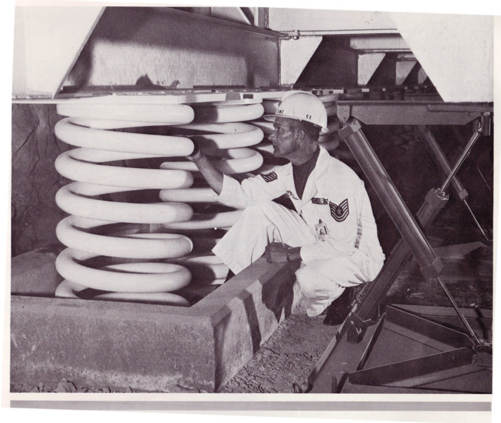
Figure 26. The buildings rested on more than 900 steel springs, meant to absorb the shock of an earthquake or nuclear explosion. Source: Henry W. Hough, NORAD Command Post: The City Inside of Cheyenne Mountain (Denver, CO: Green Mountain Press, 1970).
